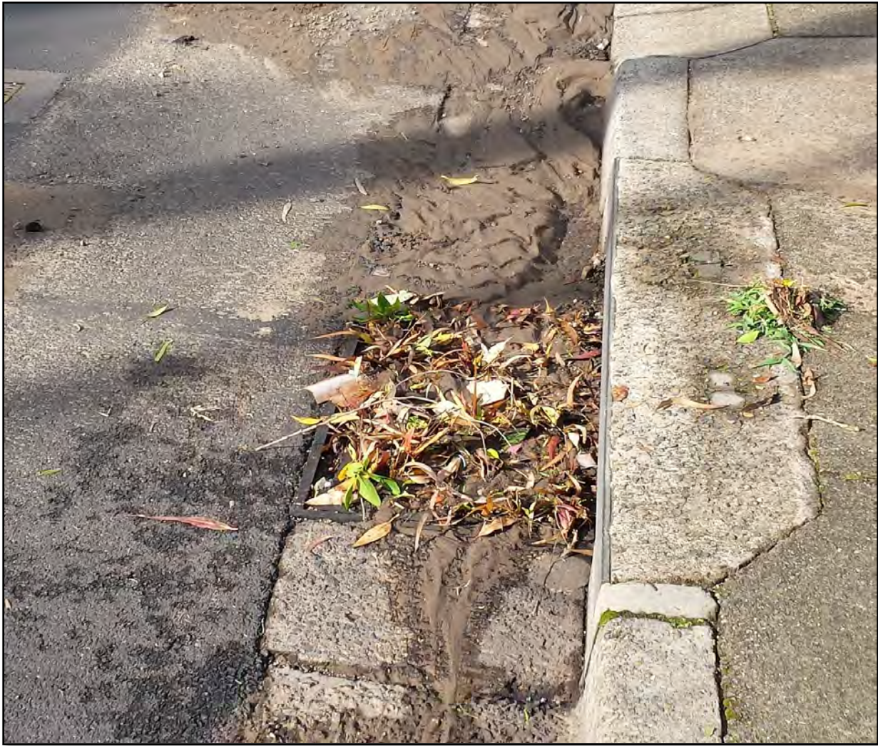
Plate 9 View showing blockage of a stormwater pit
