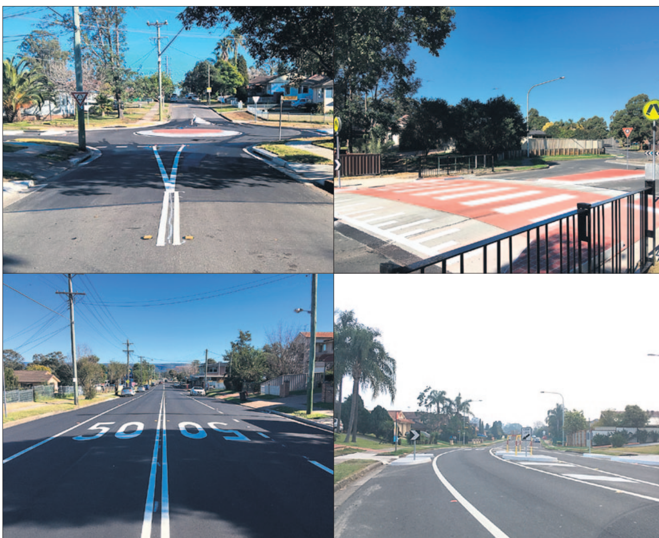
Clockwise from top left: roundabout construction, Barlow Street and Hollier Street, Cambridge Park, raised pedestrian crossing in Hindmarsh Street, Cranebrook, road reconstruction in Smith Street, South Penrith and pedestrian refuge island in Swallow Drive, Erskine Park
