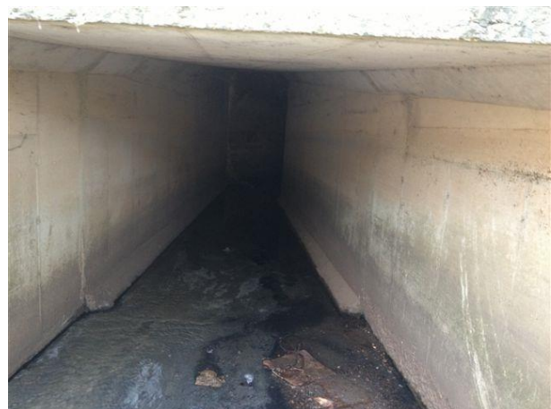
Photo 3: Hobart St conversion chamber No. 1
