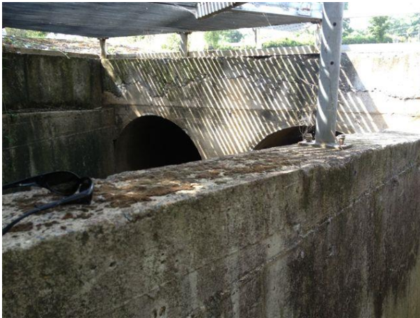
Photo 4: Hobart Street mixing chamber and inlet grate
