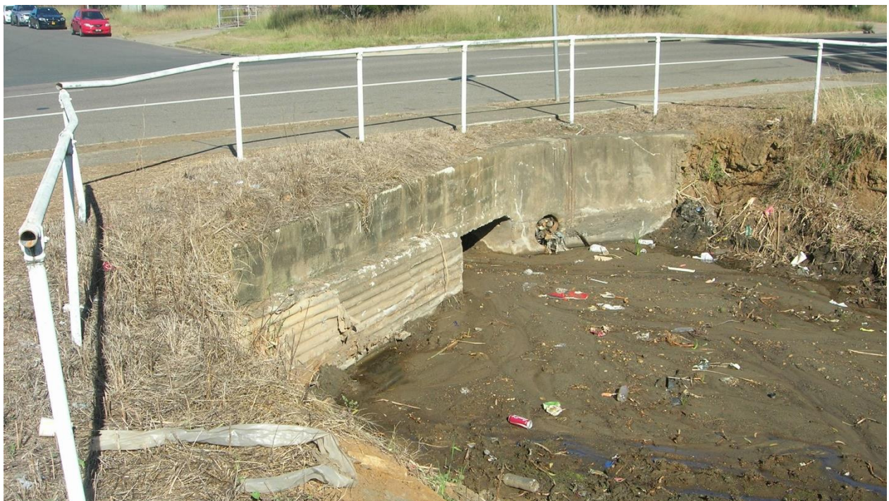
Photo 10: Eastern branch pipe outlet at Kurrajong Road after Council maintenance
