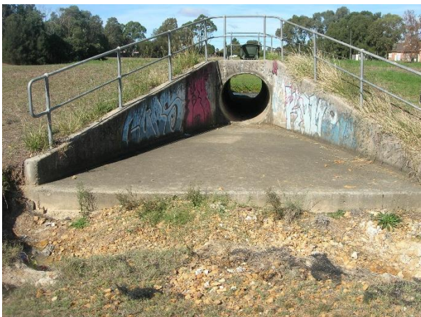
Photo 20: Control structure in Oxley Park basins
