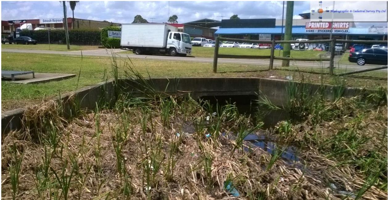
Photo 8: Outlet of trunk drainage system at Kurrajong Road
