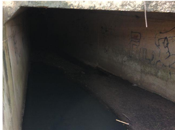
Photo 5: Hobart St conversion chamber No. 2
