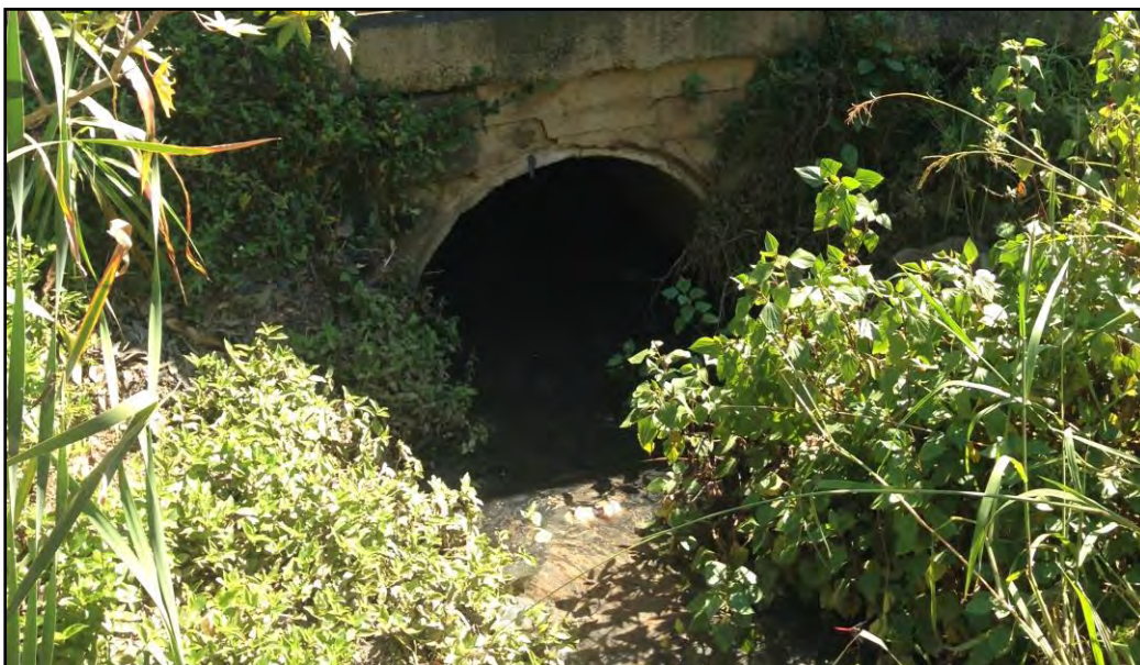
Plate 40 View looking north showing partially blocked outlet of 1.2 metre diameter pipe draining Cox Avenue area.
