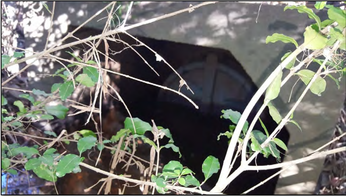
Plate 13 Photograph showing partially submerged flood gate on downstream side of Werrington Road culvert
