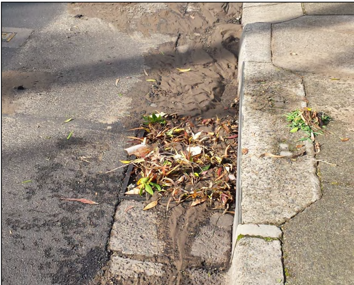
Plate 7 View showing blockage of a stormwater pit
