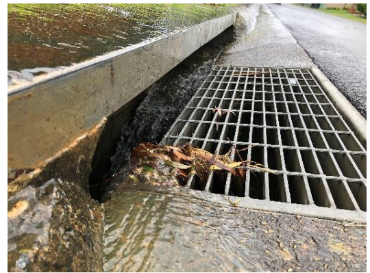
Photo: Stormwater entering the roadside kerb
