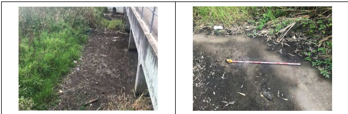
Plate 9 and 10. Showing significant modifications and disturbances to northern side of Claremont Creek, including concrete apron (close-up), bank modifications and introduced plant species, facing east.
