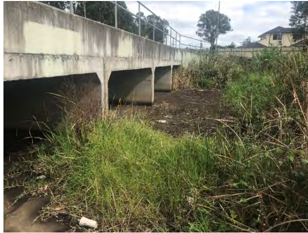
Plate 1. Significant modifications and disturbance to Claremont Creek, facing west.
