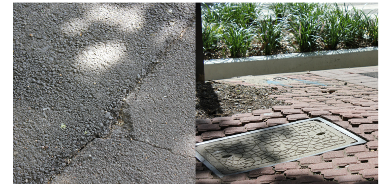
Damage to existing footpath area from weather and trees roots.
