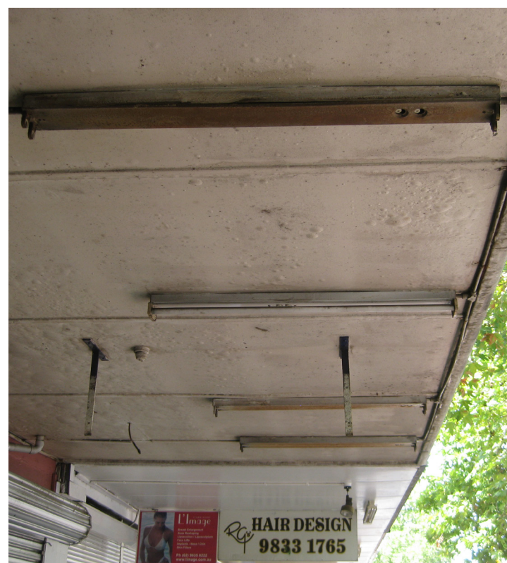
Example of various under awning lighting fixtures.
